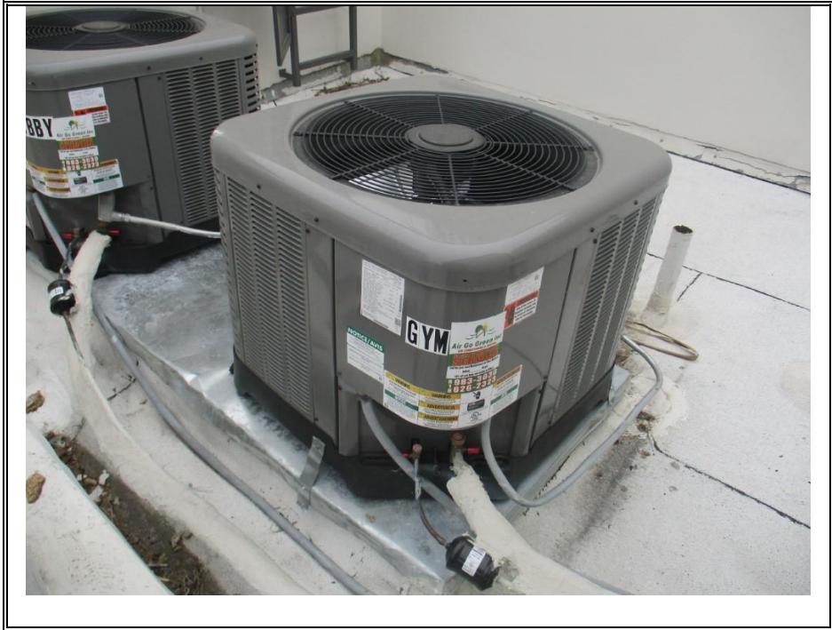
AIR CONDITIONING-CONDENSORS (TYPICAL)
