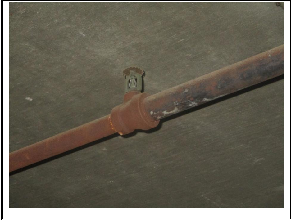
FIRE SPRINKLERS (TYPICAL)
