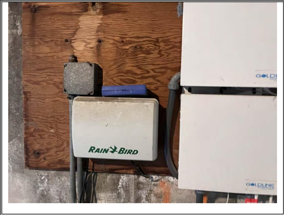
IRRIGATION CONTROLLERS (TYPICAL)
