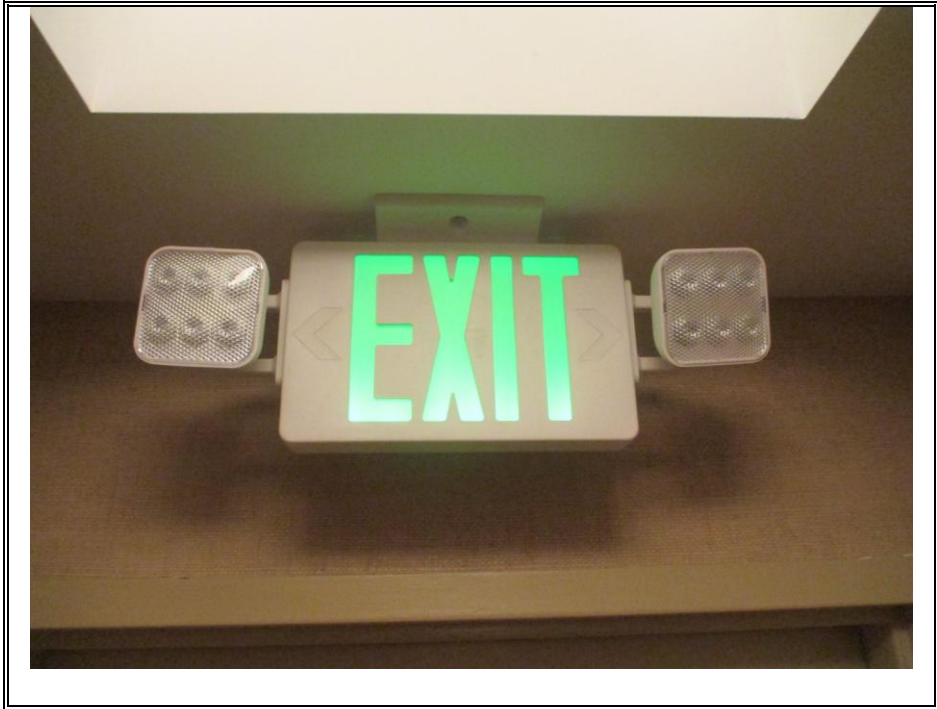
LIGHTING-EXIT SIGNS (TYPICAL)
