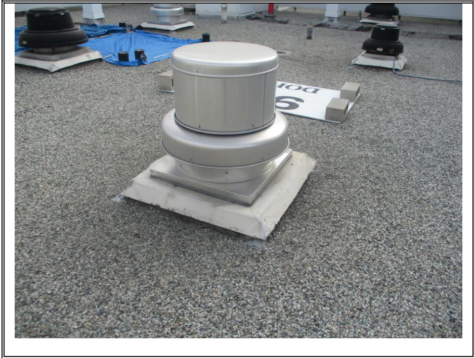
EXHAUST FANS-INTERIORS (TYPICAL)
