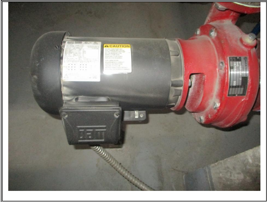
CIRCULATION PUMPS (TYPICAL)
