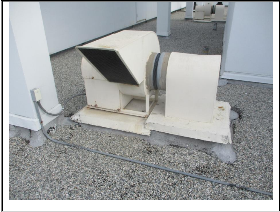
EXHAUST FANS-GARAGE (TYPICAL)
